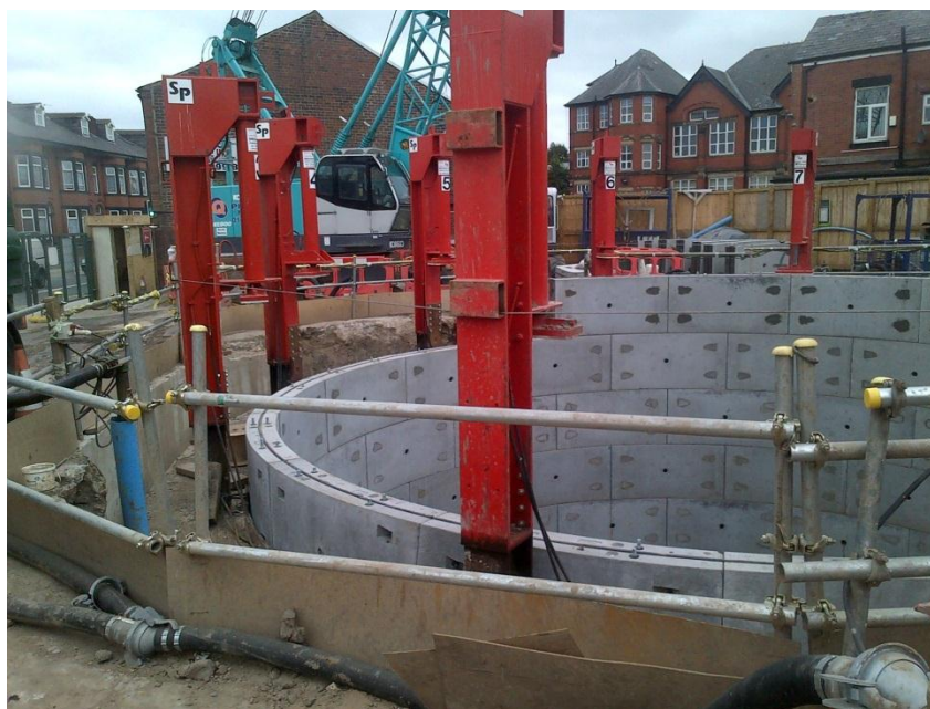
Improvements to sewer and drainage infrastructure at Park Road, Rochdale (United Utilities 2013)
